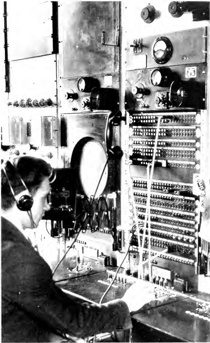
FIGURE 5. ONE OF THE GENERAL CONTROL MEN AT NEW YORK TAKING PART IN A SWITCHING OPERATION WHICH MAY INVOLVE THE COORDINATED WORK OF A NUMBER OF OTHER EXPERTS AT WIDELY SCATTERED POINTS
